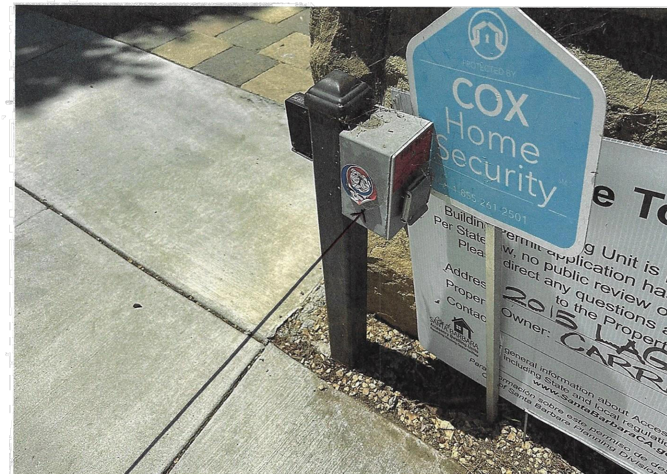
FIRE ACCESS LOCK ACTIVATOR
