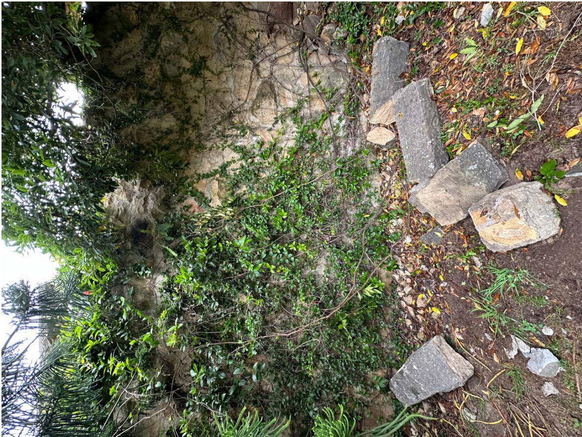
Lateral stones from the top of the wall, now 15 feet below in the barranca. Each large one weighs hundreds of pounds.
