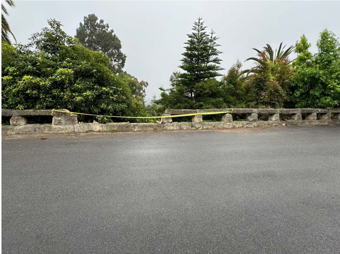
Damaged section at 1615 Lasuen Rd
