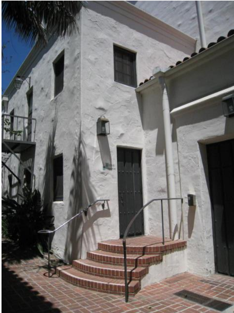
Plate 9. Green Room door showing existing steps which will be reconfigured. Facing northeast.
