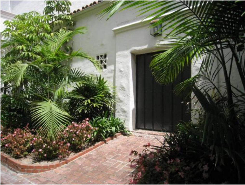
Plate 7. West exit door where stairs and landing will be added. Facing northeast.
