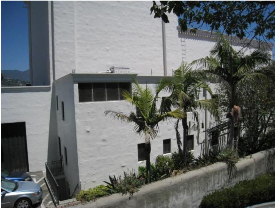
Plate 4. View from second level of parking garage of Green Room roof where added HVAC equipment will be hidden by high wall. Facing west.
