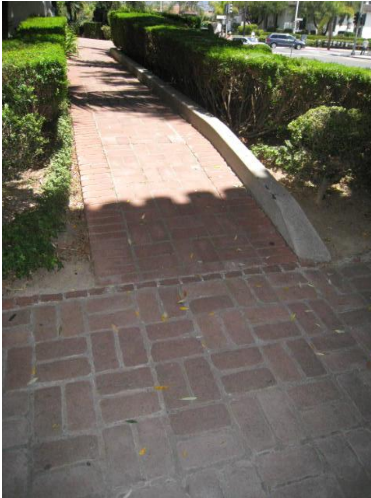
Plate 3. View of path on west side to be reconfigured for ADA access. Facing east.
