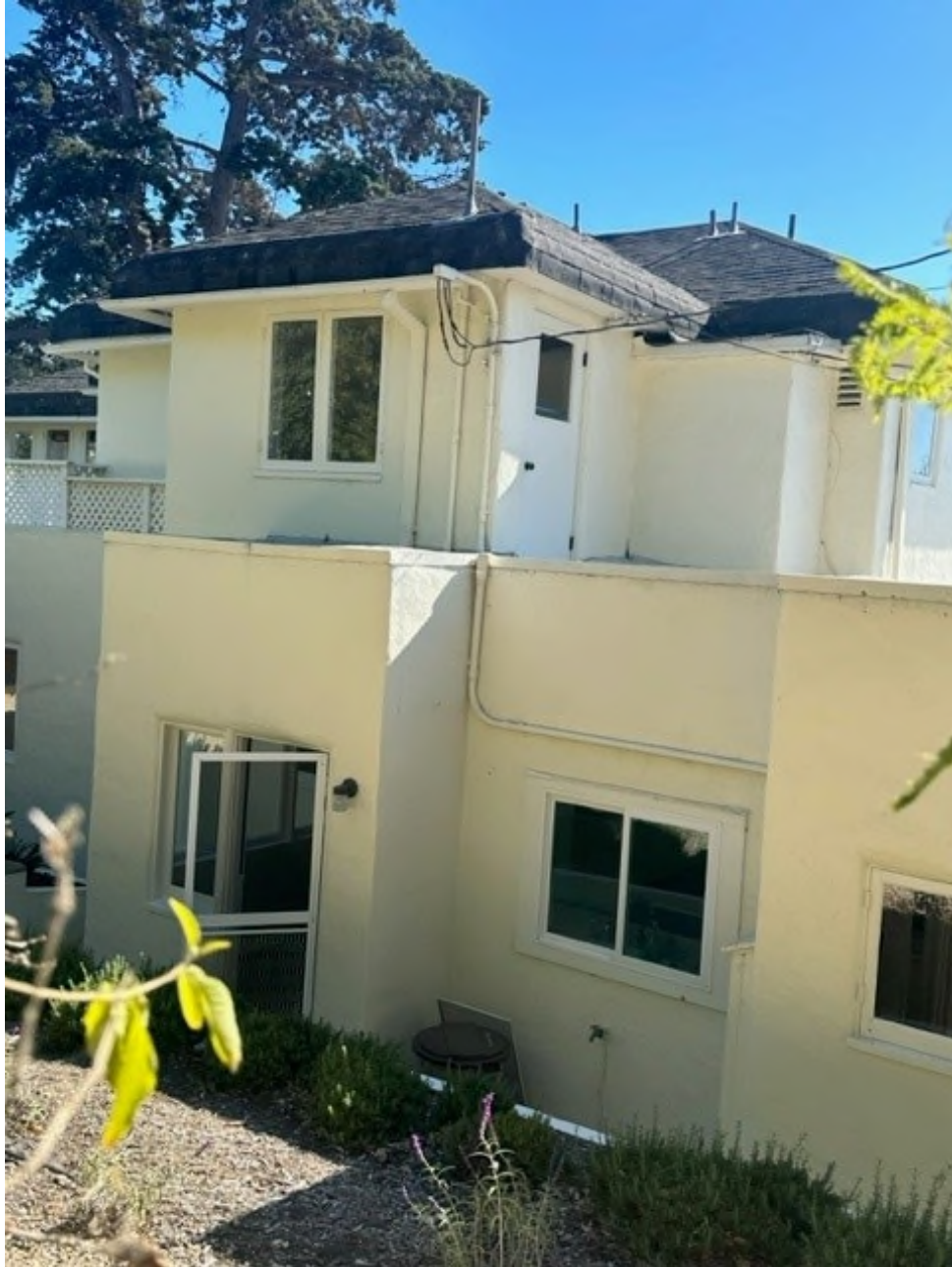
Figure 12, A partial view of the west end of the south elevation, looking southeast
