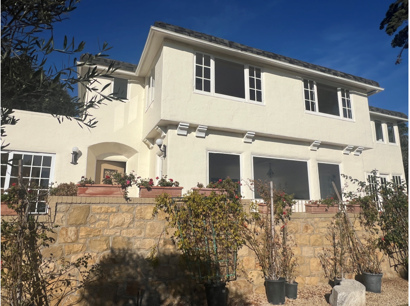
Figure 7, The central section, and west end of the south elevation, looking northeast
