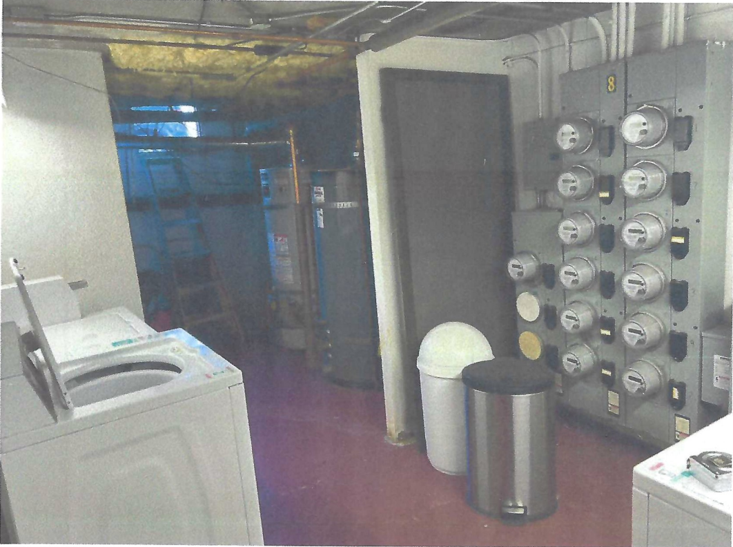
Utility Room for new HP Water Heaters
