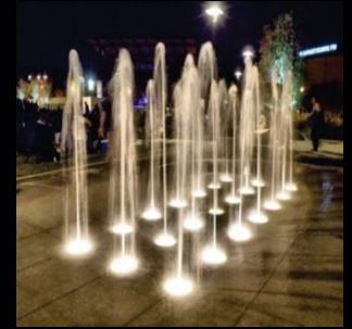
SPLASH PAD LIGHTING
