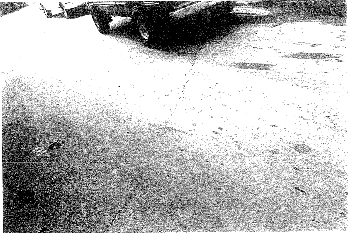
Photo 7 Pavement crack near 444 Conejo Road, 1/13/05.
