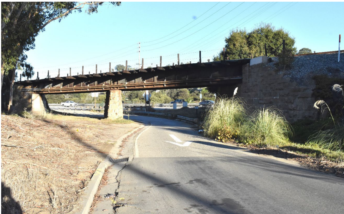
The Los Patos Way off-ramp and rail bridge, as seen from Los Patos Way south of the UPRR tracks, facing northwest.
