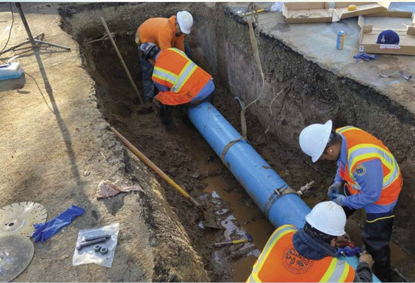
Water main pipelines are one of the City's largest assets and staying on pace to replace old pipelines is a priority.
